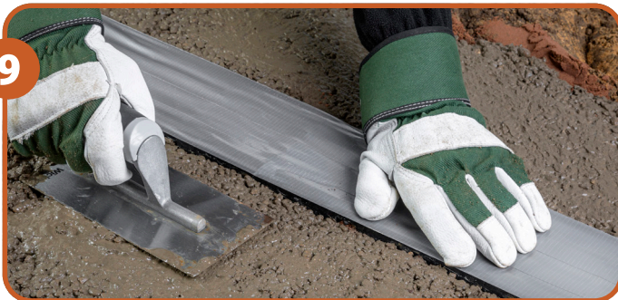
9 Pour concrete and finish 2mm above level of grate. Allow 72 hours to cure before vehicle use or removing grates.
