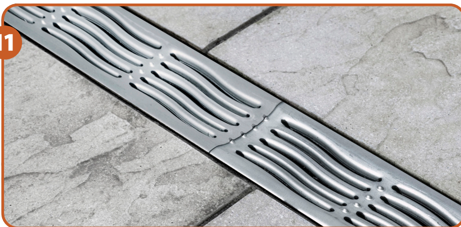
11 If installing block paving or paving slabs, support the channel (haunch) with concrete to a height which allows the depth of the block or slab to finish 2mm above the level of grate.
